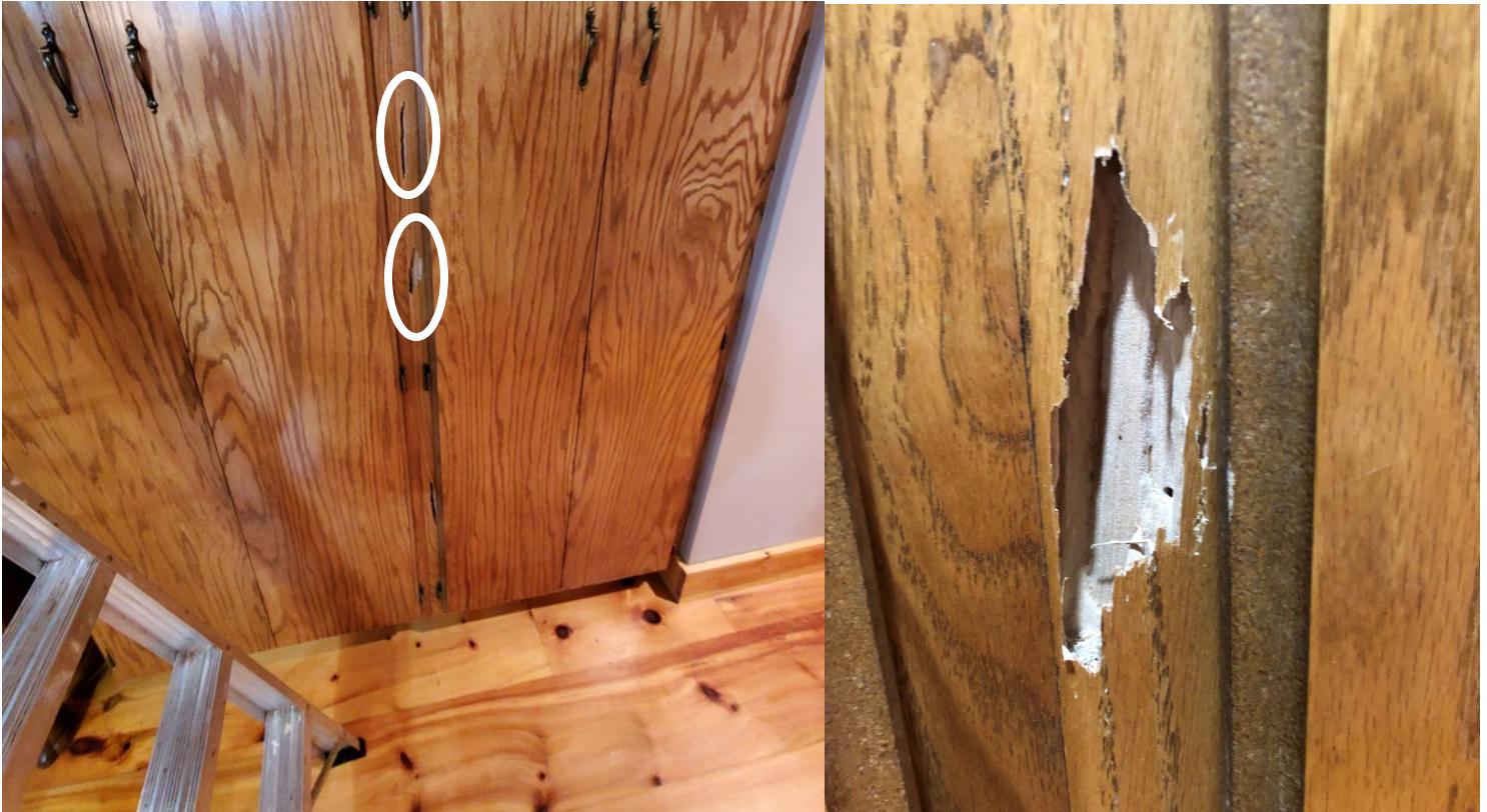
Figure 2. On the left, two drywood termite chambers circled in white were exposed when the thin wooden top layer of these kitchen cabinets was removed. Credit: John Cook. On the right is a close-up of these chambers. Credit: Karen Vail
