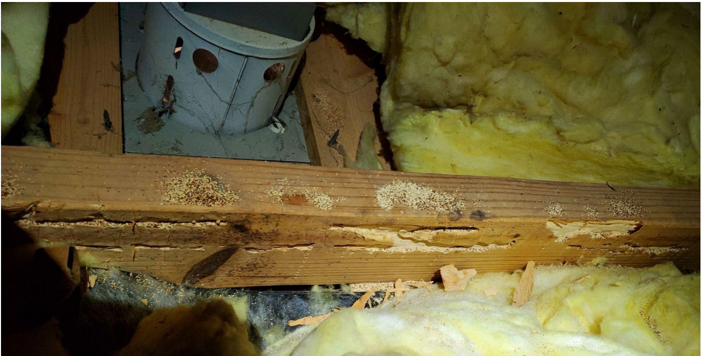
Figure 8. A pocketknife easily removed the thin wood hiding the termite chamber. Drywood termites leave a thin layer of wood to protect the colony in the chamber. Often the wood is puckered in these locations and serves as a clue to the termite galleries' locations. Credit: John Cook
