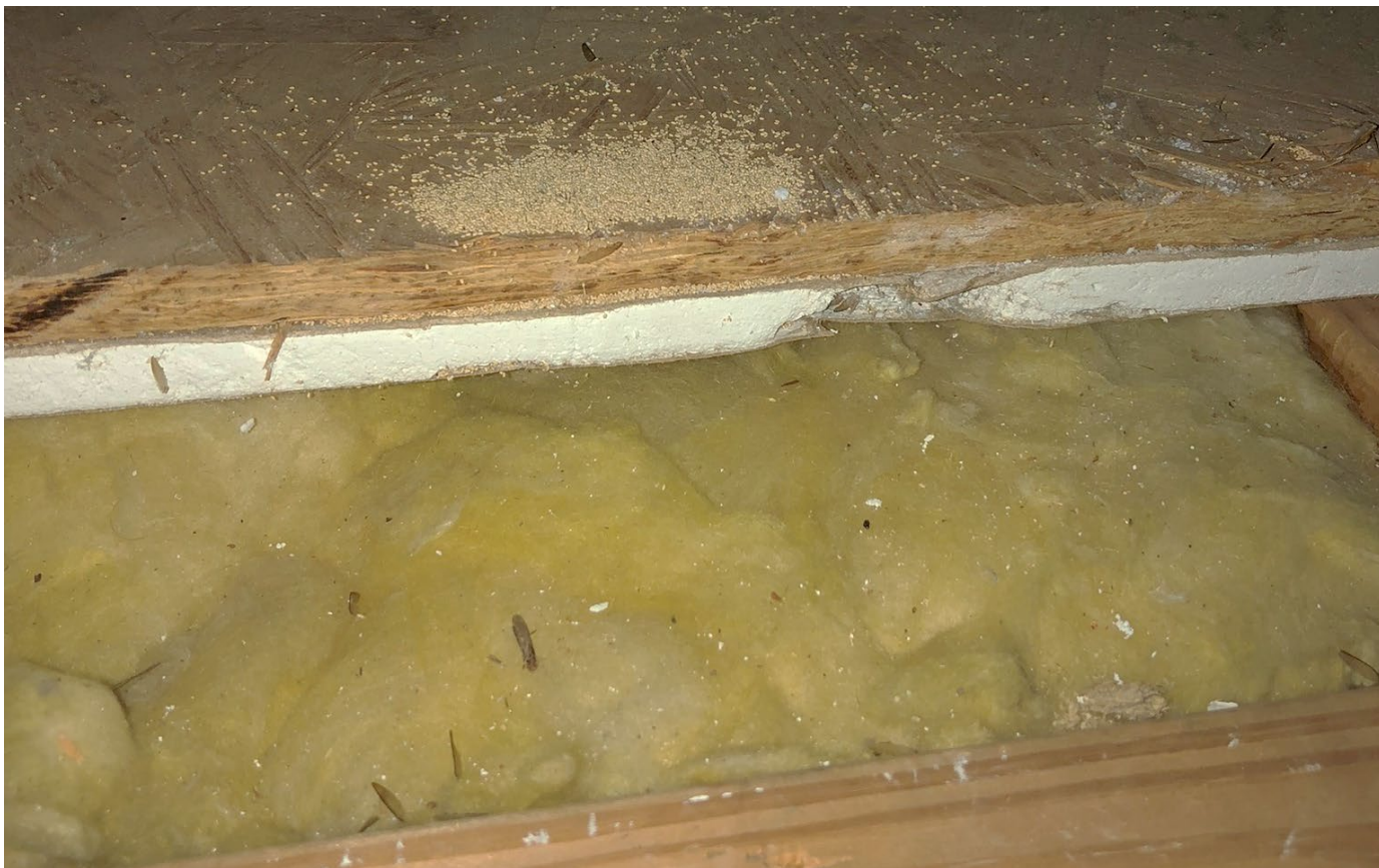
Figure 9. Two signs of drywood termites are found in this photo (1) pile of 6-sided fecal pellets and (2) swarmer wings. The pile of pellets in the photo is on top of the attic access panel so there was a colony at the very edge of the attic just feet away from those cabinets. No drywood colonies were found above the rafters. Credit: Karen Vail
