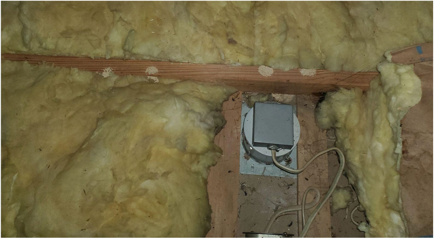
Figure 7. Piles of drywood termite 6-sided fecal pellets piled high on the attic floor joists. Normally, the fecal pellets fall to the ground, but the insulation on the sides of the board prevented the termites from creating a side gallery opening. Credit: John Cook
